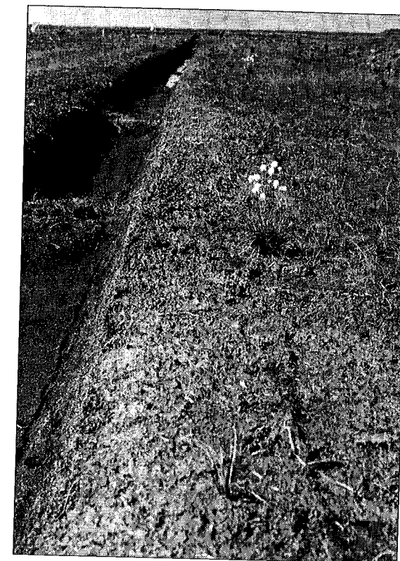
Fig. 3 Blocked drainage ditch later in the summer.
