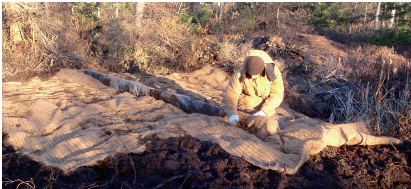
Figure 21. The installation of stabilization net at the peatland Grande plée Bleue (Québec).
