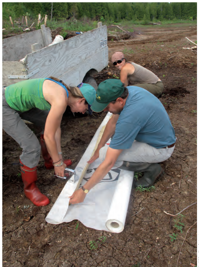
Figure 35. Installation of a geotextile at the base of a future dam at the peatland Bic – Saint-Fabien (Québec).
