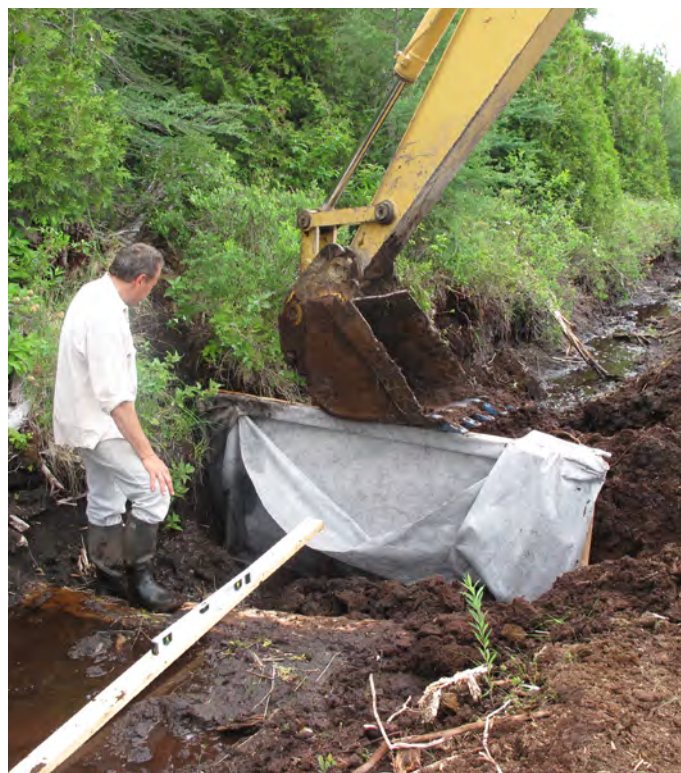
Figure 22. Installation of a wooden plank covered with a geotextile (Bic – Saint-Fabien peatland, Québec).
